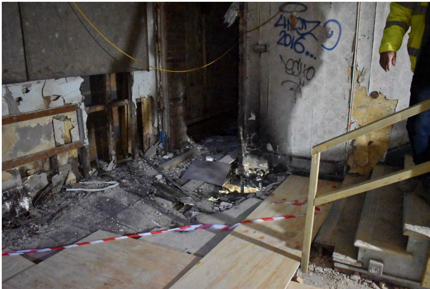
Plate 140: Main Office, Ground Floor, Room I, source of fire (December 2022, facing NE)
