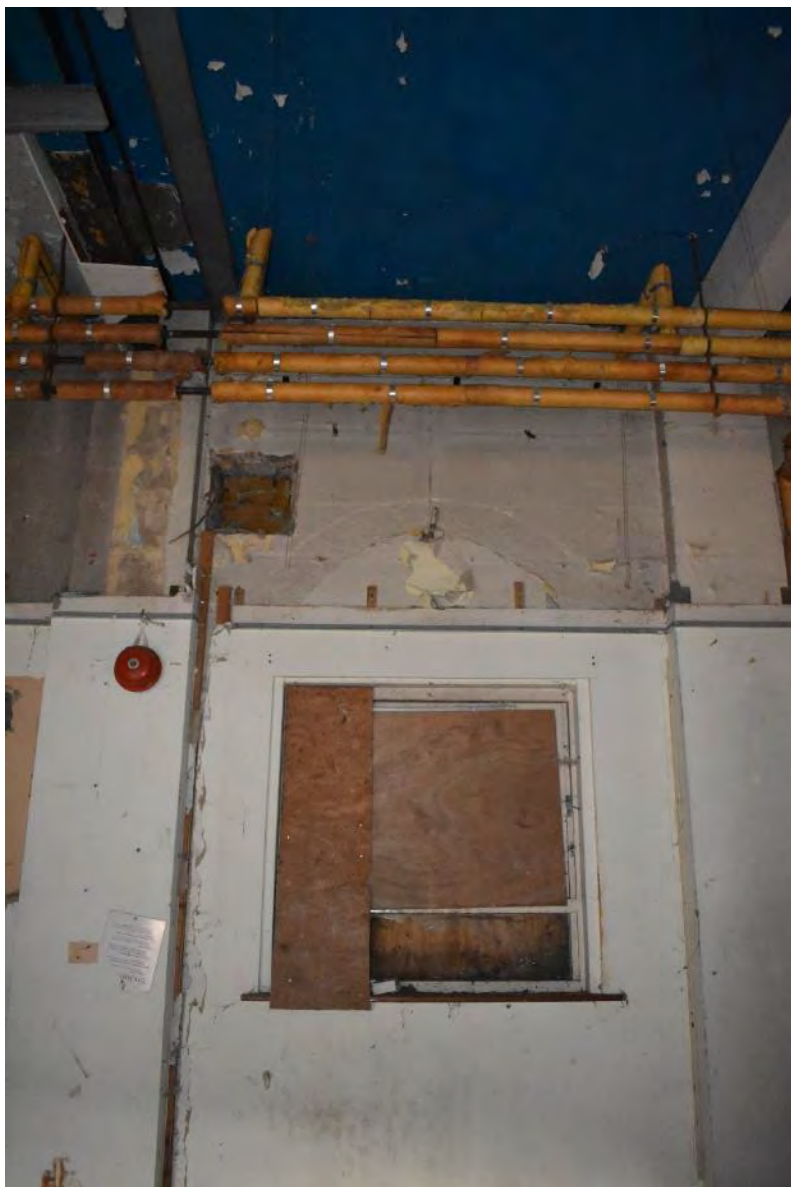
Plate 133: Ground Floor close up of altered windows (December 2022)
