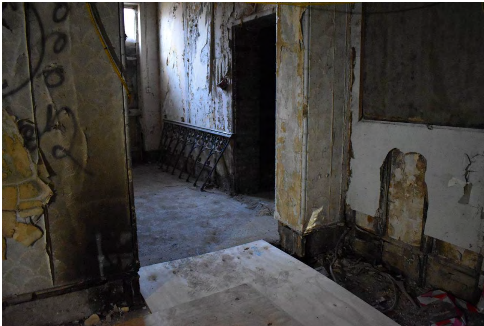
Plate 141: Main Office, Ground Floor, Room I looking towards Room J (December 2022 facing NW).
