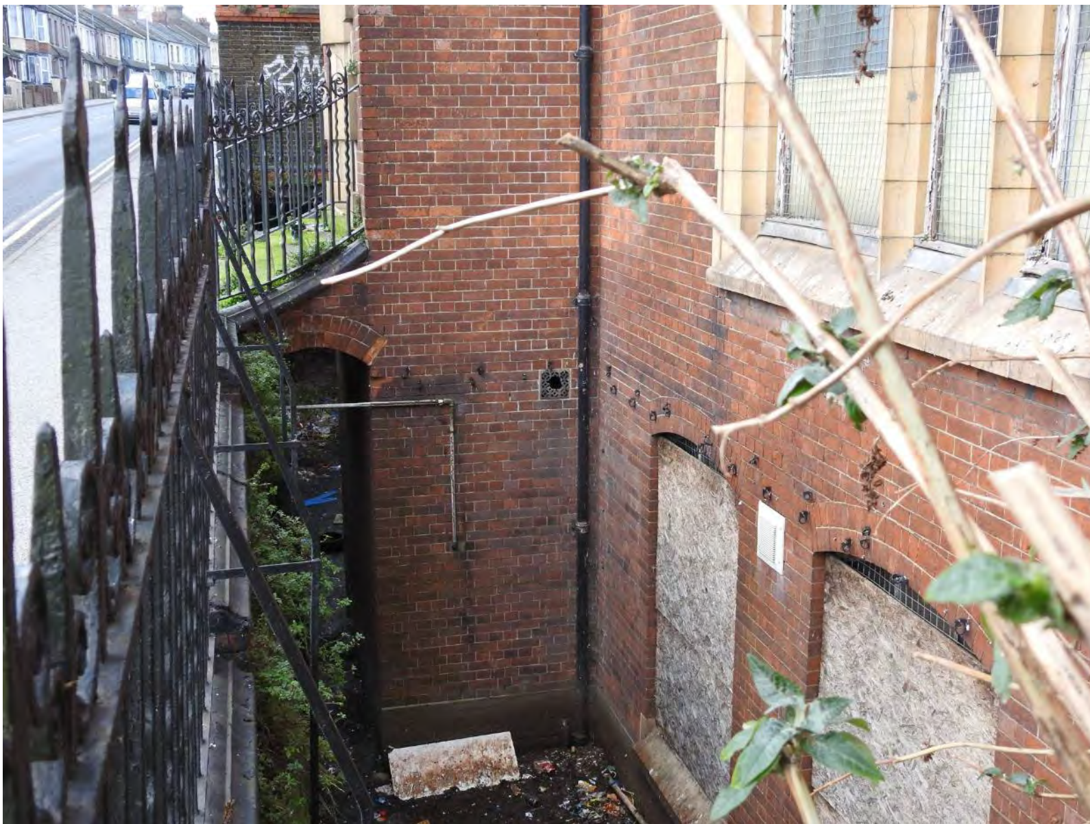
Plate 35: View of basement level southern side of the office at the eastern end (December 2020)
