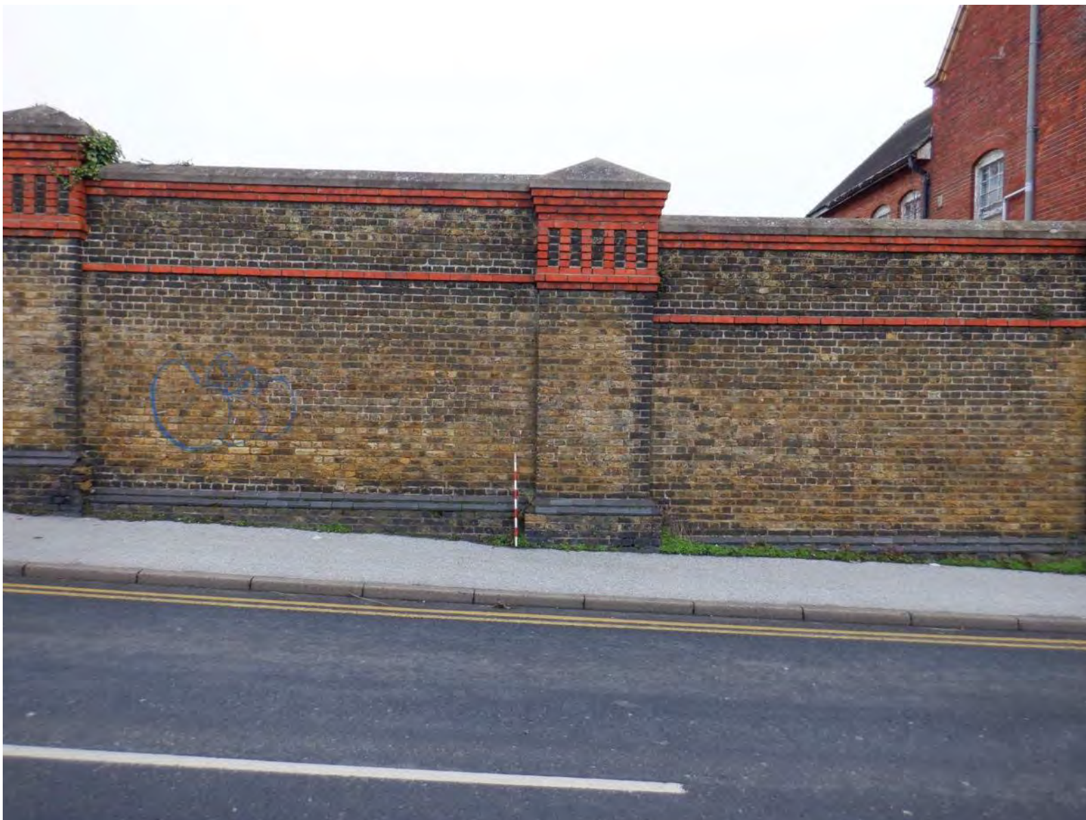
Plate 45: Southern western wall, scale 1m (August 2021 facing N)
