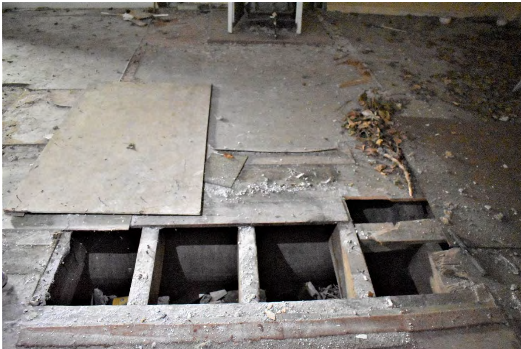
Plate 131: Remains of a 2m stretch of mains gas pipe underneath the ground floor.
