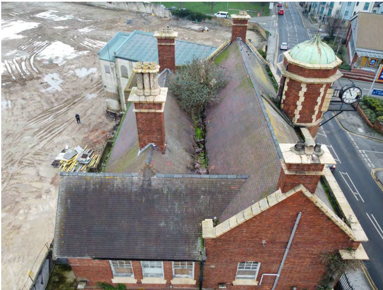
Plate 25: Aerial view of the roof from the western end (December 2020 facing NNE)
