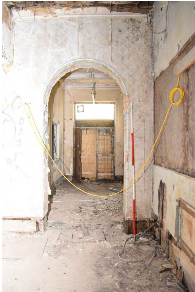
Plate 88: View towards side entrance Room J from Room I (August 2021 facing W)
